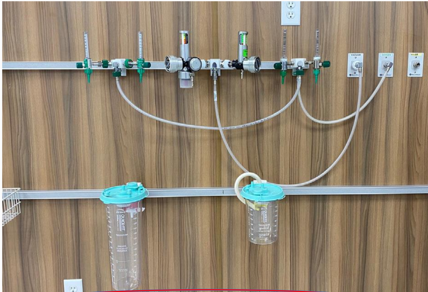
Figure 2-11: Medical Gas Expansion Rail
