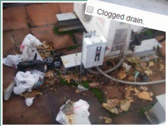
Debris on the roof.
